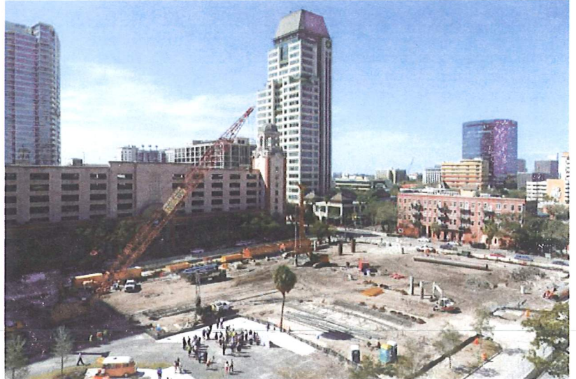
A rising population, job growth and housing demand all are pushing Florida toward becoming a $1 trillion economy within a couple years, a new report says. This photo from March shows early construction for One St. Petersburg, a 41-story, 253-unit condo tower in downtown St. Petersburg. [SCOTT KEELER | Times]
